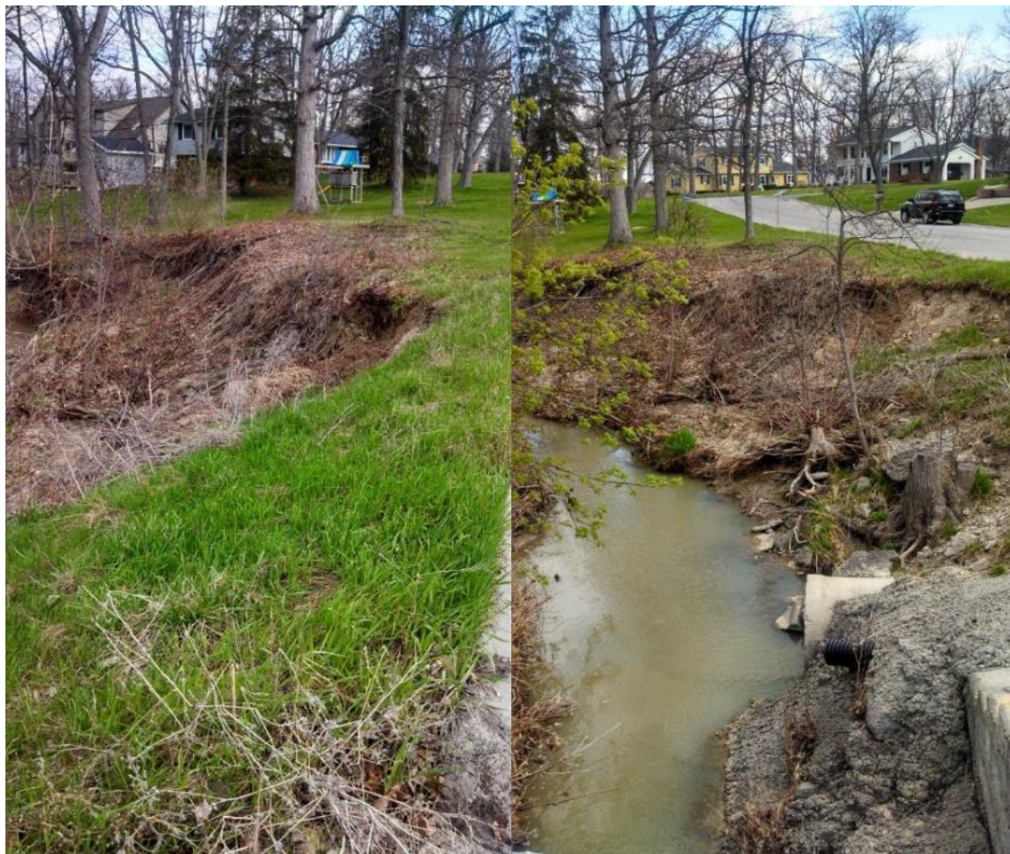
Figure 14. Preston Run bank erosion problems
