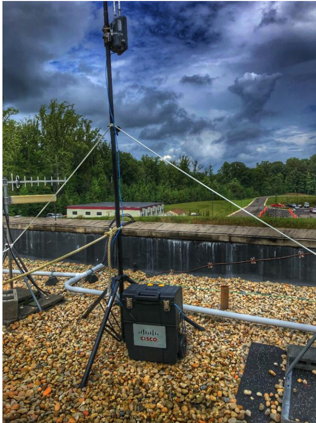
Roof-top deployment of a Cisco LoRaWAN gateway utilizing autonomous power and LTE uplink.
